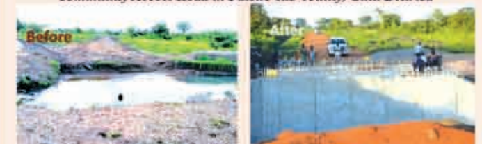
(Left) excavated area for construction of a box culvert foundation. (Right) Ongoing construction of a box culvert along Arut central - Laminto (13.8km) Climate Resilient Community Access Road in Paicho sub county, Gulu District.
