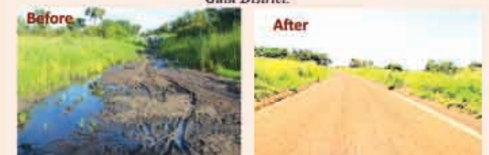
(Left) Labilo A-Labilo B before the construction and (Right) Constructed Labilo A-Labilo B Climate Resilient Community Access Road in Lagoro sub county, Kitgum
