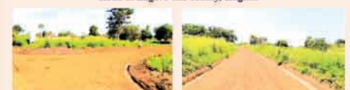
Cross section of some of the constructed Community Access Roads in the project area to enhance transportation of commodities from production areas to the market
